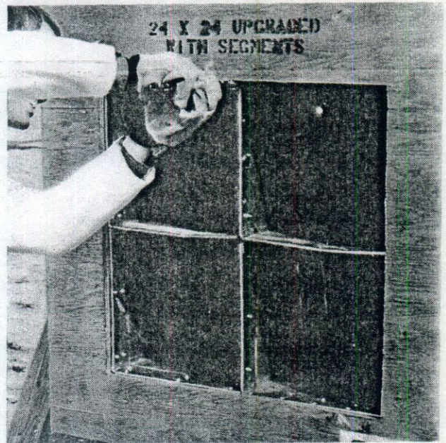
Figure 8-5b. Segmented Duct Upgrade Attack with Hand Metal Cutters
